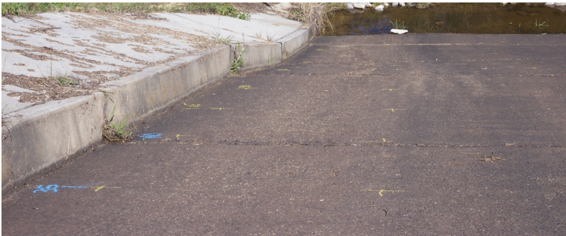
Fig. 6. Spillway Slab Showing Distortion of Concrete
